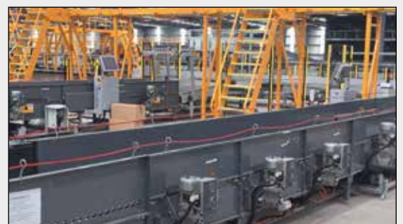
BCS solution for Toll IPEC facility Melbourne
