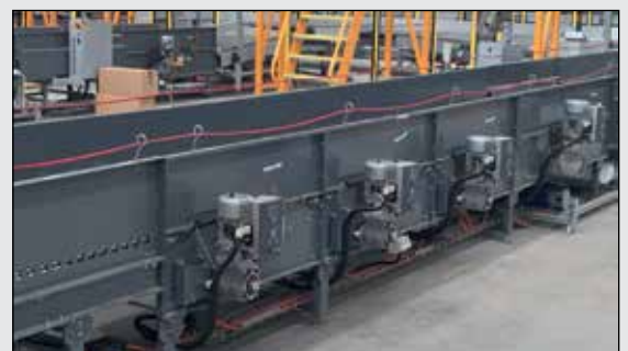
BCS solution for Toll IPEC facility Melbourne, Australia
