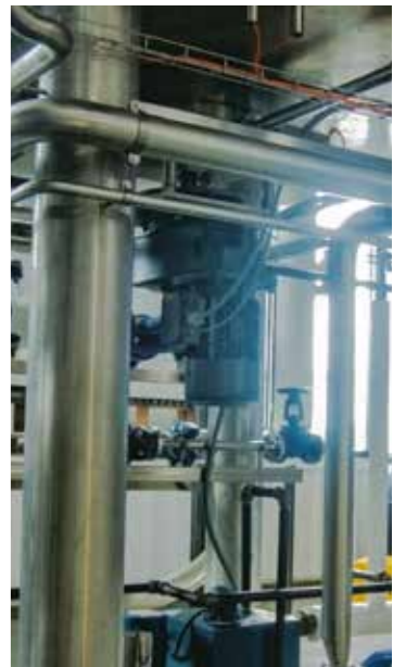
A 5 hp Parallel mounted CLINCHER™ powers the rake in the Mash Tun.
